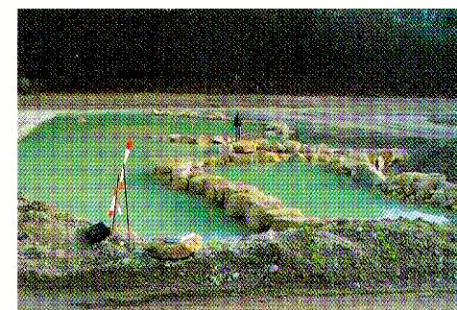
Ground ramp under construction: the staggered structure consisting of bars and pools is clearly recognisable. The base consisting of stones measuring 40 to 60 centimetres under the large stone blocks is also clearly visible.
